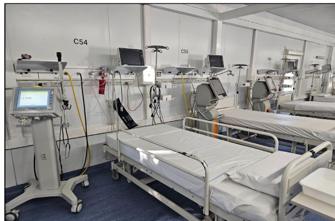
FIGURE 12. Equipment and facilities-related equipment installed in a critical care unit, MHS No. 9—Almirante Brown, Buenos Aires.
