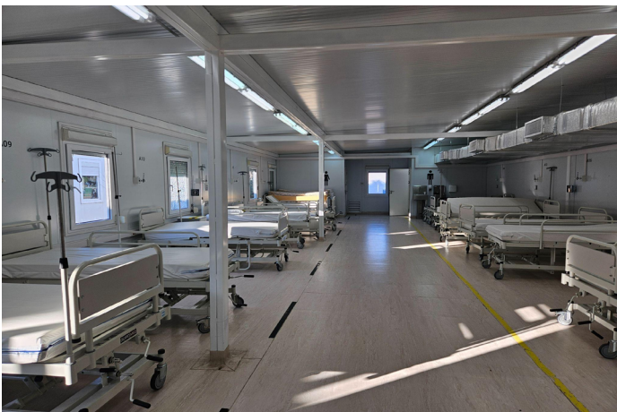
FIGURE 16. Equipment and facilities-related equipment installed in a hospitalization room, MHS No. 9—Almirante Brown, Buenos Aires.
