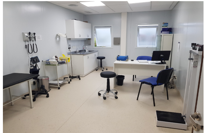
FIGURE 17. Equipment installed in an emergency office, MHS No. 28—Exaltación de la Cruz, Buenos Aires.
