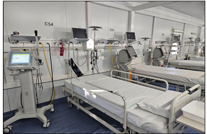
FIGURE 12. Equipment and facilities-related equipment installed in a critical care unit, MHS No. 9—Almirante Brown, Buenos Aires.
