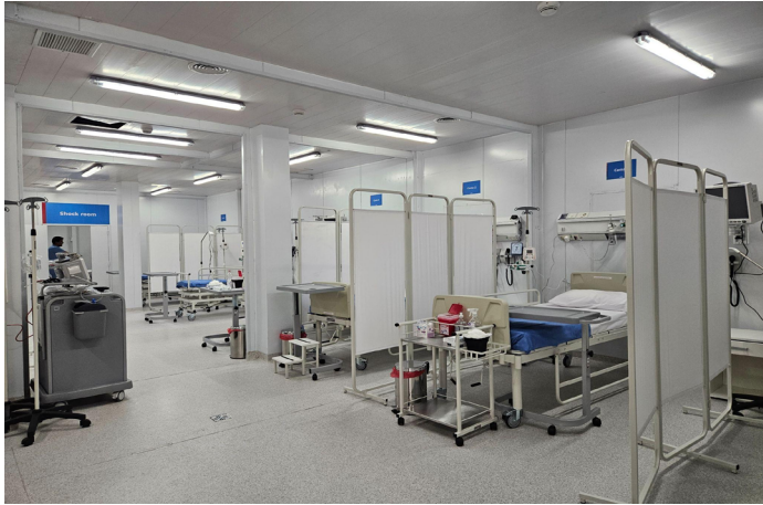
FIGURE 15. Equipment and facilities-related equipment installed in an observation sector, MHS San Jorge, Córdoba.
